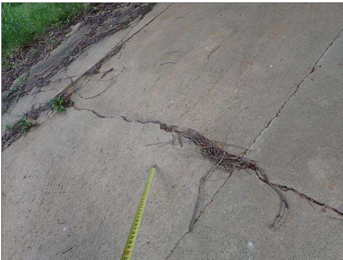
end bent 2 slope protection, transverse crack (up to 1 inch wide) with settlement (up to 1.5 inches)
