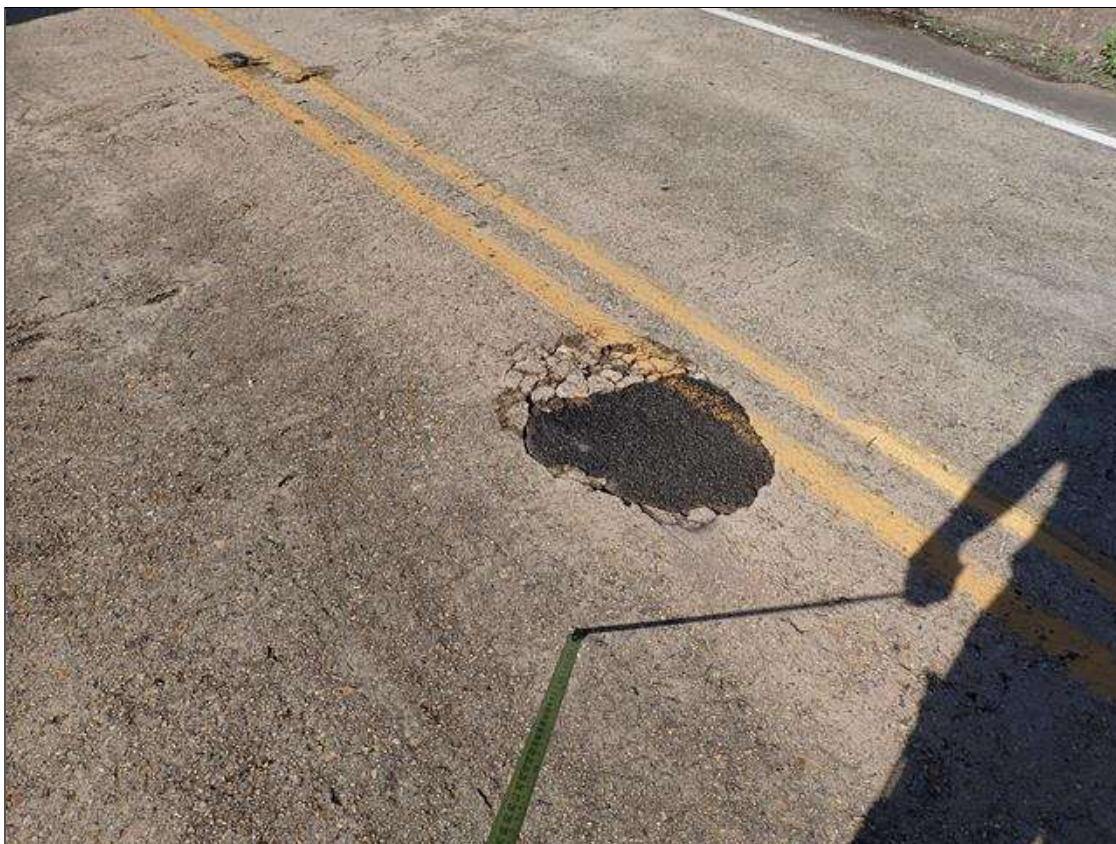
Span 1 Deck: throughout top of deck, asphalt patches (up to 2 foot diameter)
