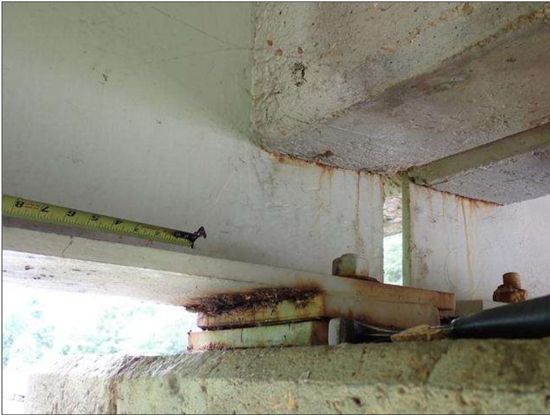
Span 1 Beam 1: at bent 1, web adjacent to diaphragm, painted over section loss (9/16 inch average remaining x 4 inch x 1 inch) with corrosion reinitiated; bottom flange, rust scale
