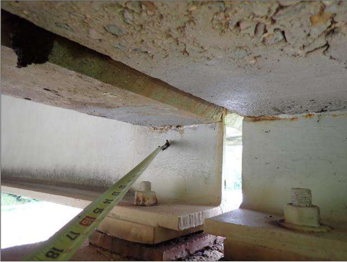
Span 2 Beam 4: at bent 1, web adjacent to diaphragm, painted over section loss (1/2 inch average remaining x 10 inch x 1 inch) with corrosion reinitiated
