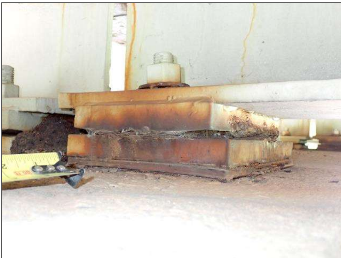
Span 2 Beam 2 - Far Bearing 2: RUST SCALE/PACK RUST ON THE BEARING PLATE.
