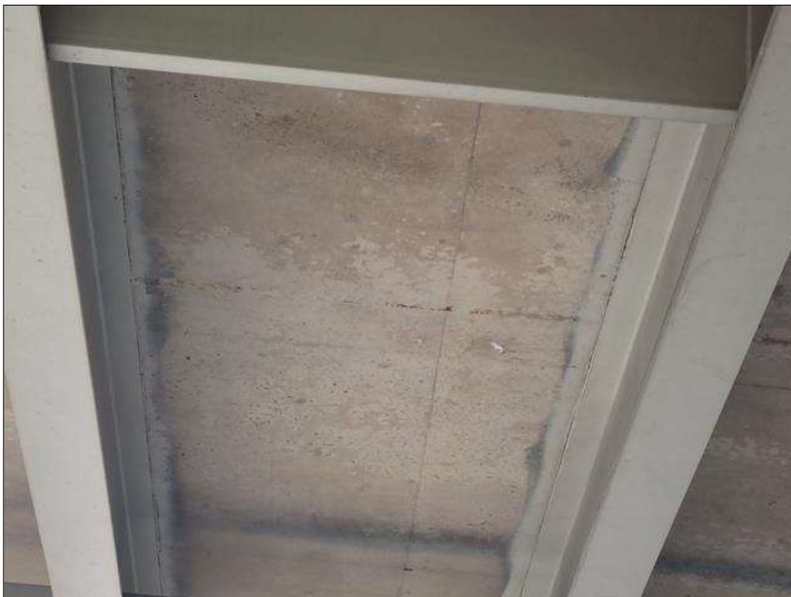
Span 3 Deck: SPAN 3 BOTTOM OF DECK HAS HAIRLINE MAP CRACKING WITH SOME EFFLORESCENCE IN ALL BAYS; BOTH OVERHANGS, TRANSVERSE CRACKS (HAIRLINE X FULL WIDTH), SOME WITH EFFLORESCENCE
