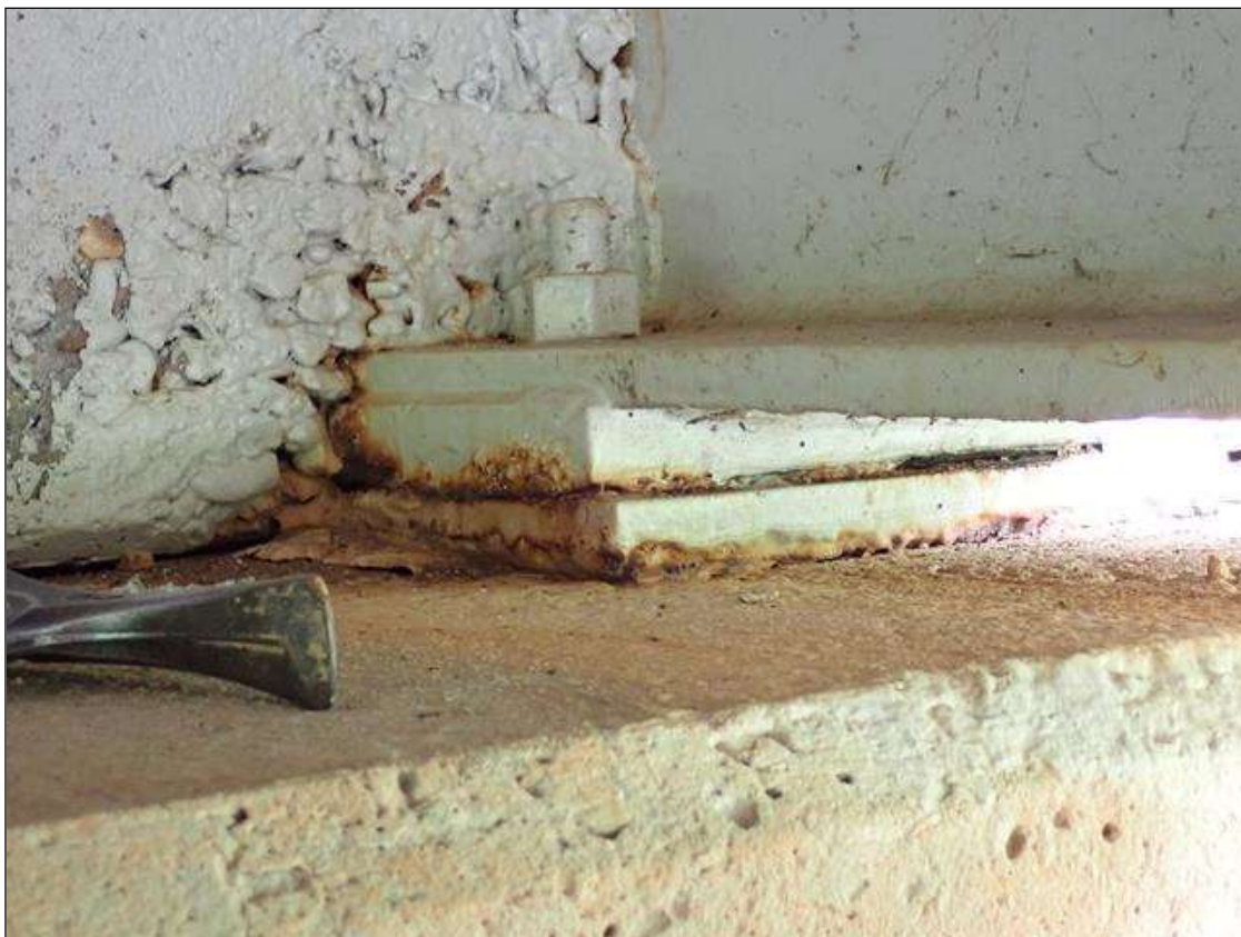
Span 1 Beam 1 - Near Bearing 1: painted over section loss (up to 3/16 inch deep) with corrosion reinitiated
