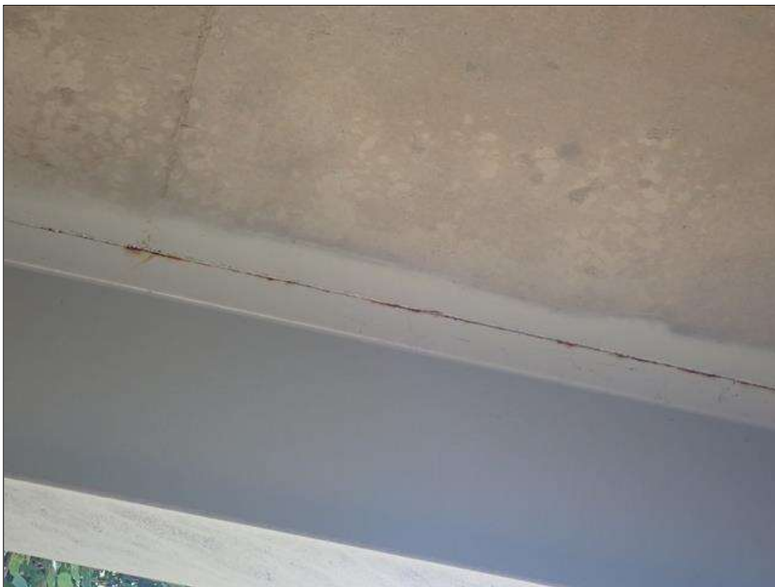
Span 4 Beam 4: along the edge of the top flange, near bent 3, surface rust
