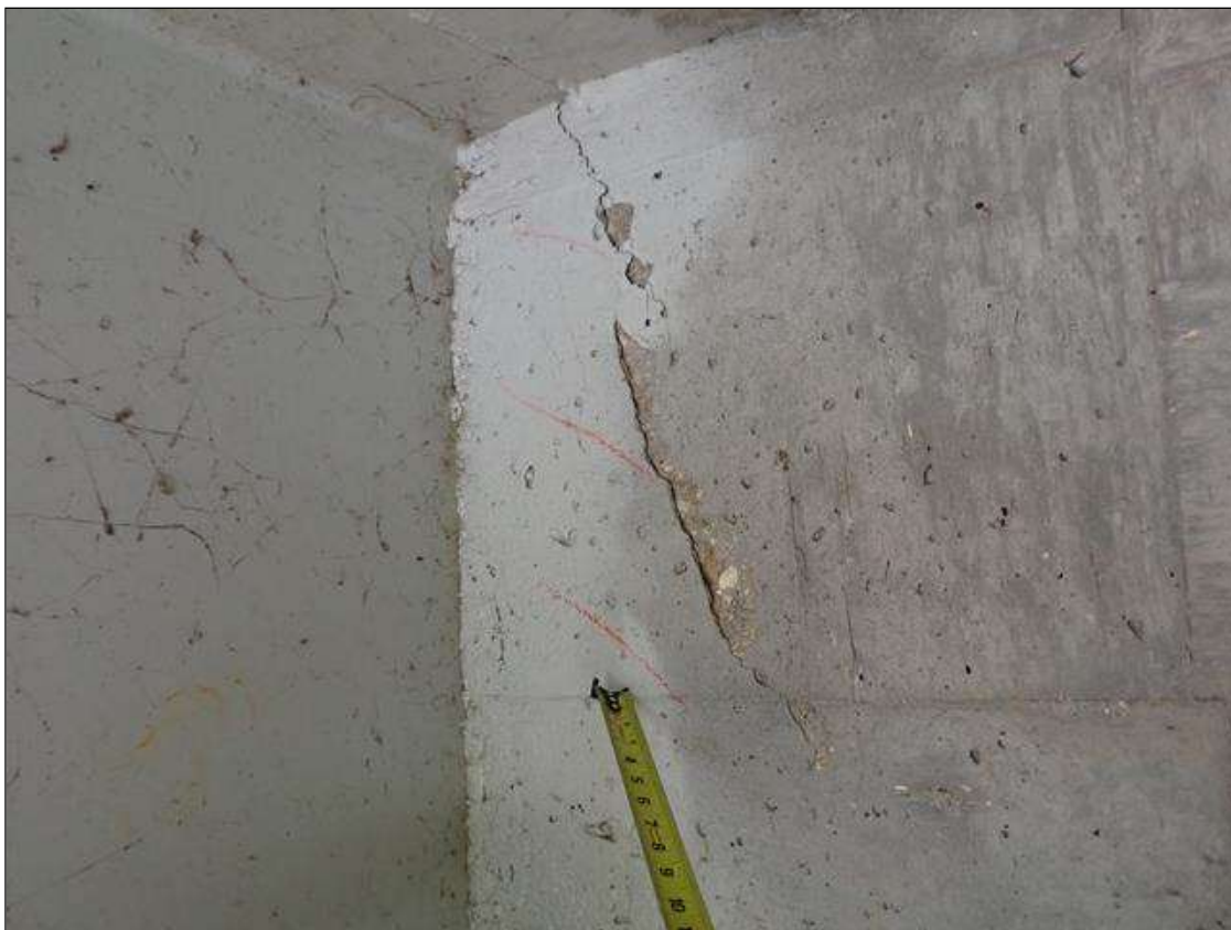
End Bent 1 Abutment: adjacent to all beams, delaminations/spalls [up to 2 feet x 13 inch x 1/2 inch deep]
