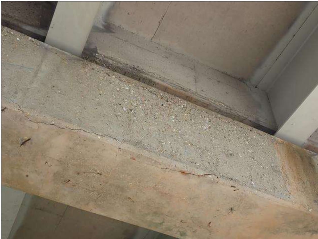
Bent 3 Cap 1: (PAR) along the length of the cap, delaminations/spalls (up to full length x 10 inches high x 1.5 inch deep) with cracks (up to 1/8 inch) with some rust stains
