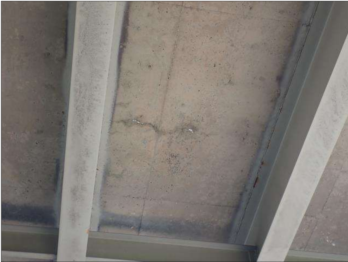
Span 2 Deck: SPAN 2 BOTTOM OF DECK HAS hairline map cracking, some WITH EFFLORESCENCE IN ALL BAYS; BOTH OVERHANGS, TRANSVERSE CRACKS (HAIRLINE X FULL WIDTH), SOME WITH EFFLORESCENCE
