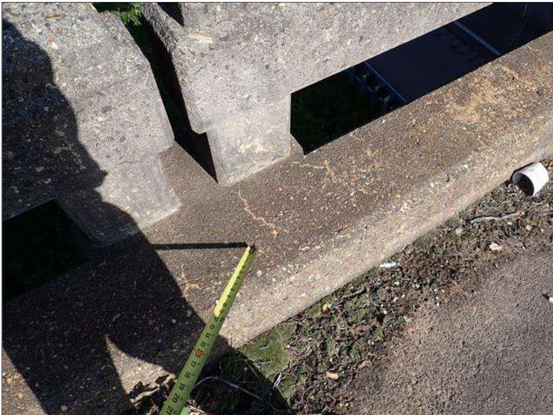
Span 1 Left Bridge Rail: along the curb, areas of map cracks (hairline) at random
