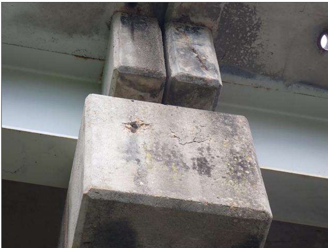
Bent 1 Cap 1: RIGHT END OF CAP HAS A SPALL AREA 5 INCH X 5 INCH X 3/4 INCH DEEP WITH REBAR EXPOSED AND 6 INCH DIAMETER DELAMINATION.
