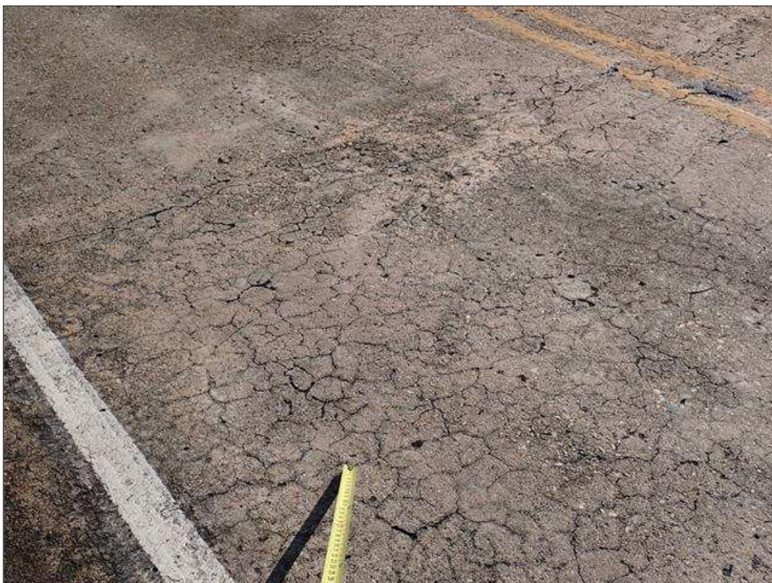
Span 1 Deck: throughout top of deck, map cracks (up to 1/16 inch) and transverse cracks (up to 1/16 inch x 15 feet) at random
