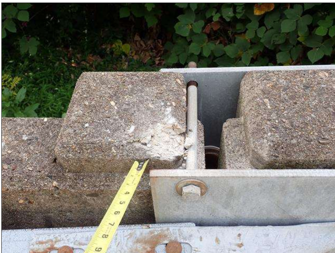
Span 4 Right Bridge Rail: top of rail post 7, spall (4 inch diameter x 1 inch deep)
