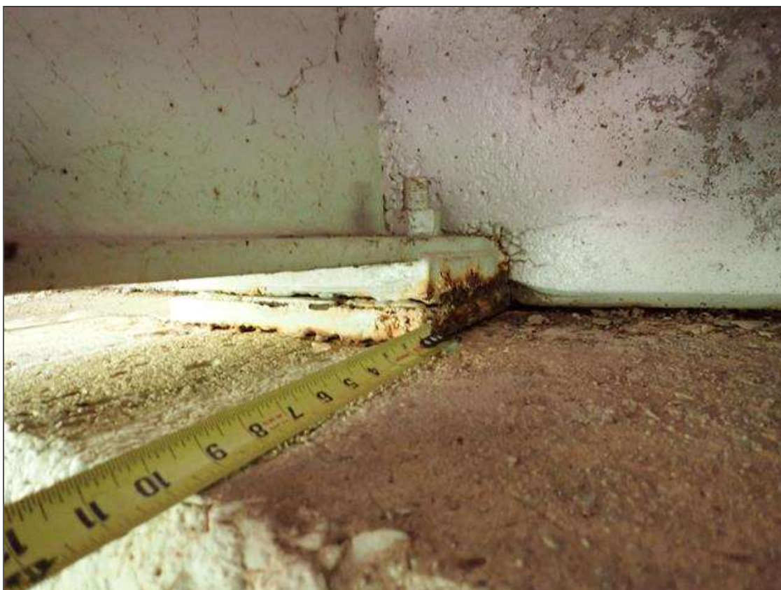
Span 4 Beam 1 - Far Bearing 1: rust scale
