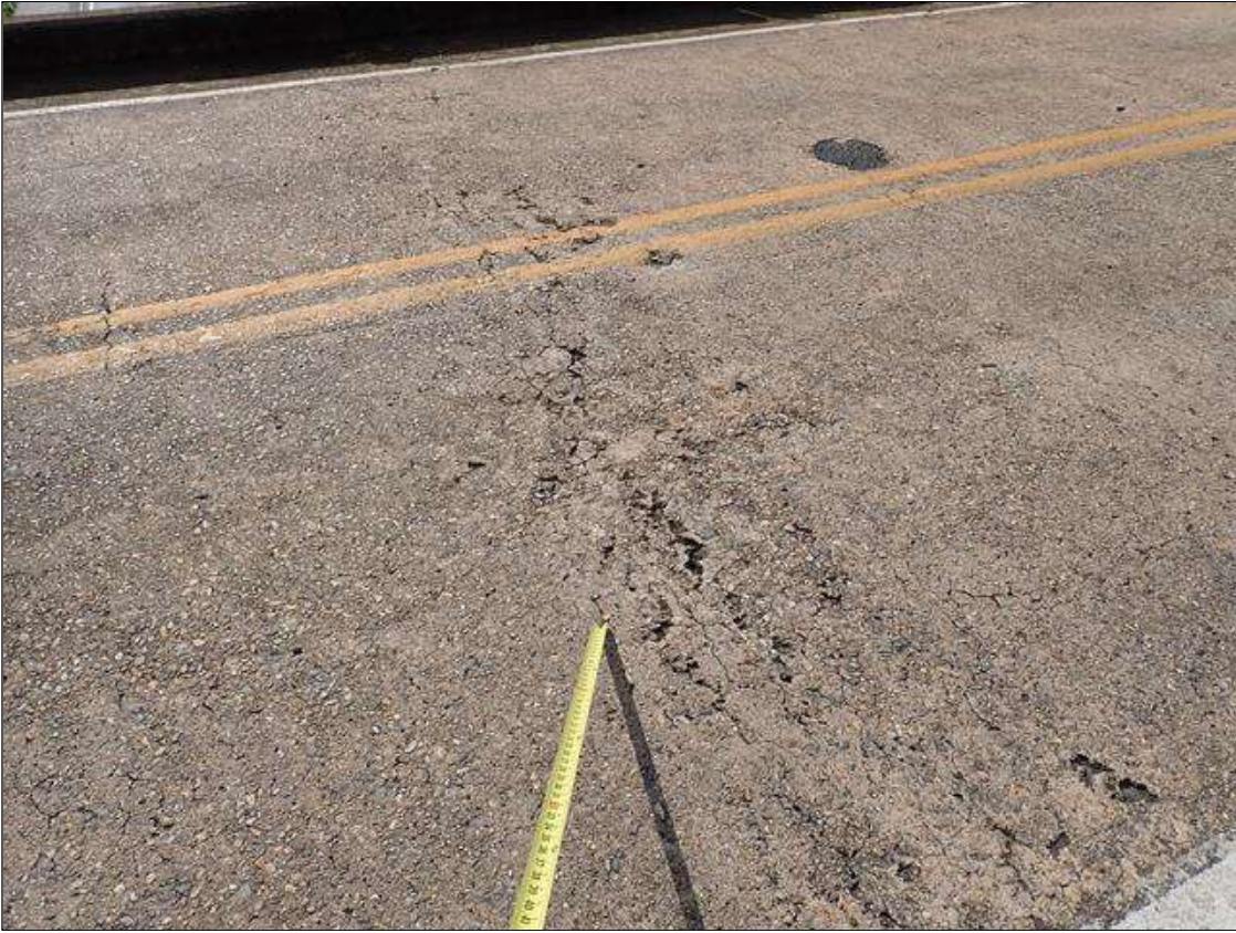
Span 3 Deck: throughout top of deck, scattered delaminations/spalls (up to 2 foot x 1 foot x 1 inch deep)
