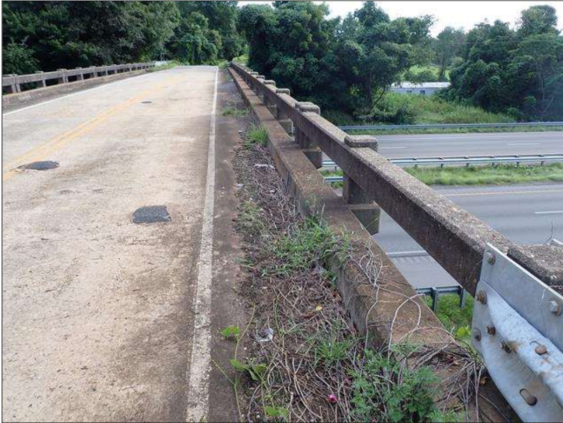
along the curblines, areas of debris accumulation (up to 2 feet wide x 3 inches high) with vegetation, partially obstructing deck drains
