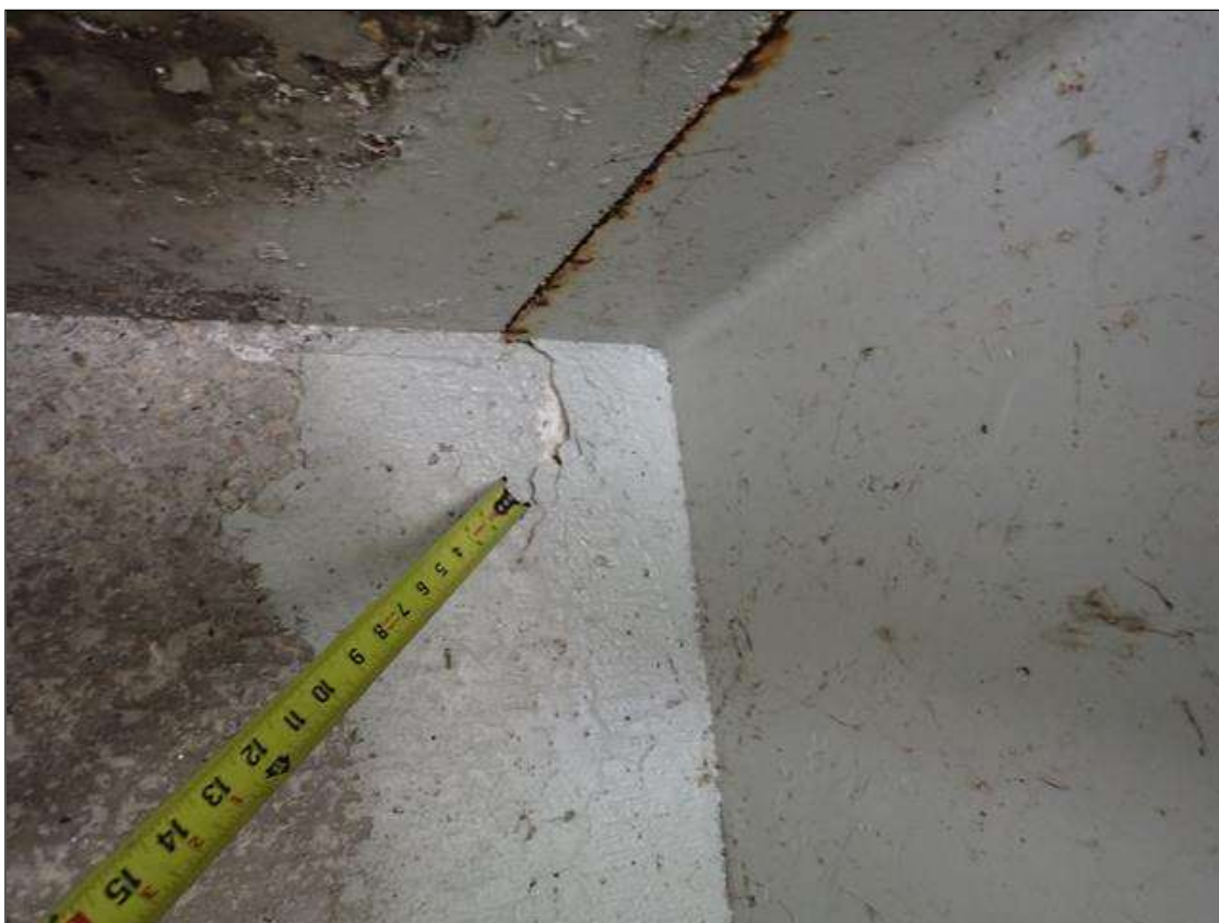
End Bent 2 Abutment: in bay 1, adjacent to bay 2, delamination (9 inch x 5 inch)
