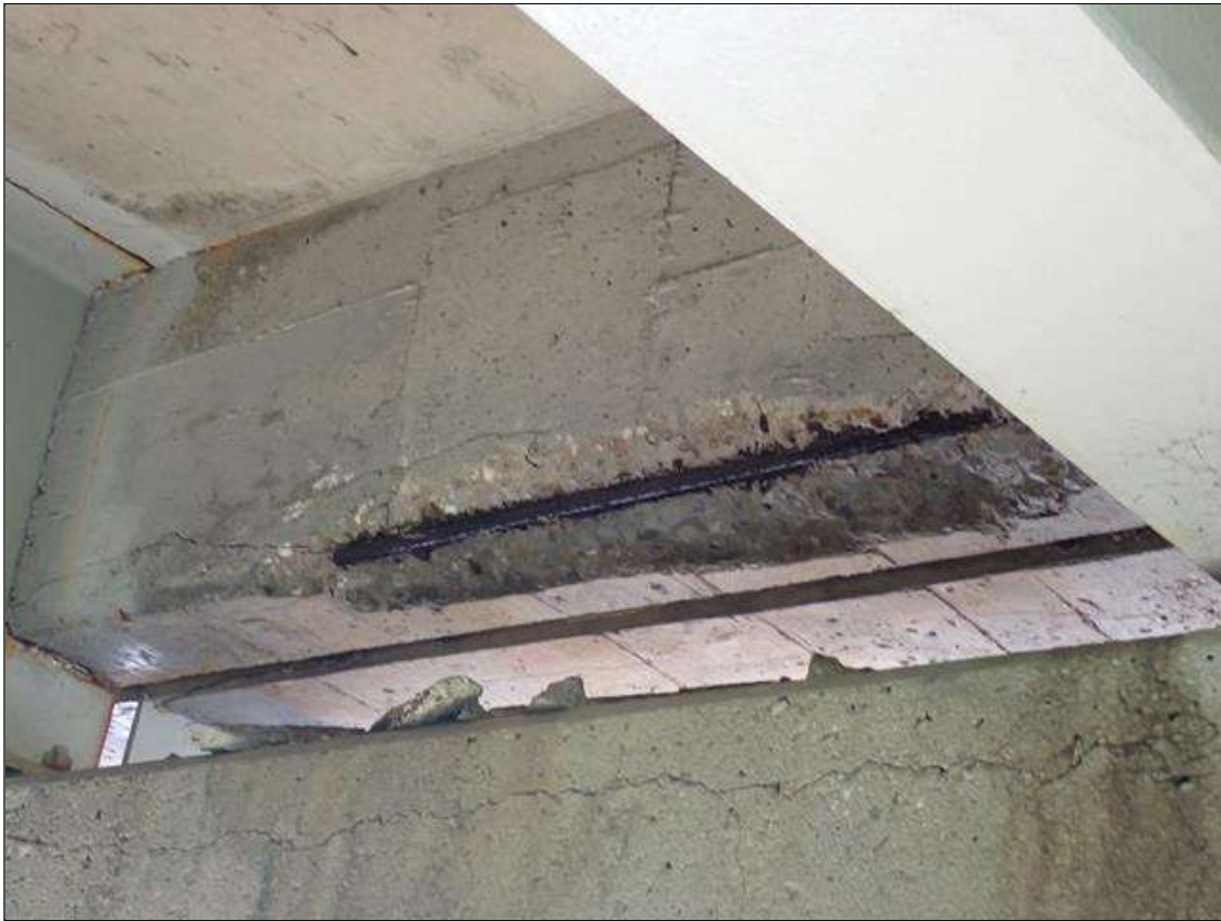
Span 4 Deck: at bent 3, end diaphragm in all bays, spalls/delaminations (up to full bay width x 10 inches x 2.5 inches deep) with exposed rusted rebar, with associated cracks (up to 1/16 inch)
