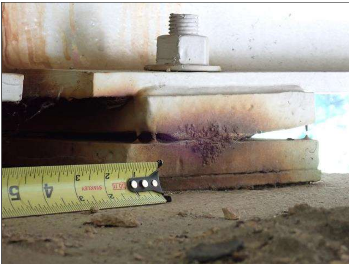
Span 3 Beam 2 - Far Bearing 2: SPAN 3 BEAM 2 FAR BEARING HAS SURFACE RUST/PACK RUST ON BEARING PLATE.
