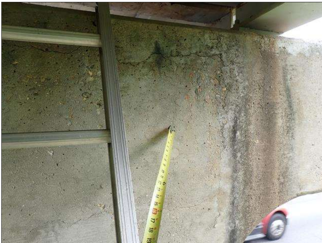
Bent 1 Cap 1: along the length of the cap, delaminations (up to 7 feet x 6 inch) with cracks (up to 1/16 inch)
