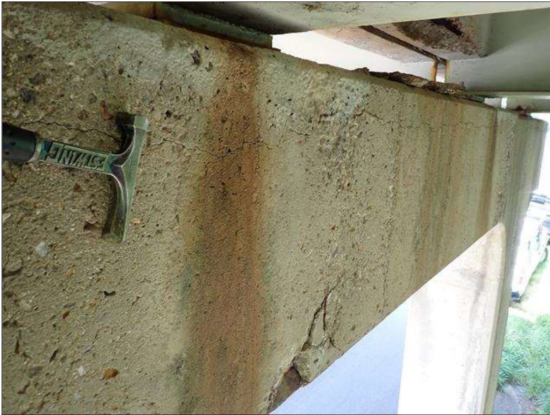
Bent 3 Cap 1: (PAR) along the length of the cap, delaminations/spalls (up to full length x 10 inches high x 1.5 inch deep) with cracks (up to 1/8 inch) with some rust stains
