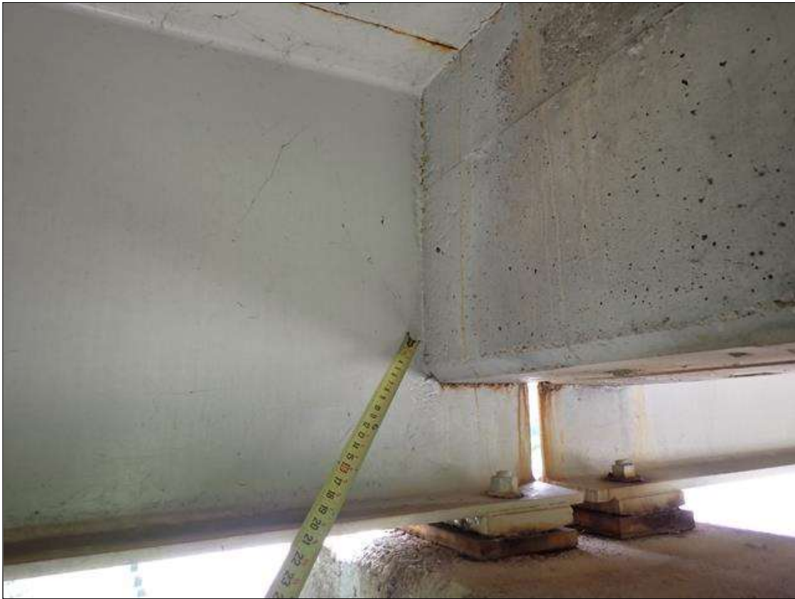
Span 4 Beam 4: at bent 3, painted over section loss: web adjacent to diaphragm (7/16 inch average remaining x 1 inch x 2 feet); lower web, painted over pitting (up to 1/16 inch deep x 1 foot) with corrosion reinitiated
