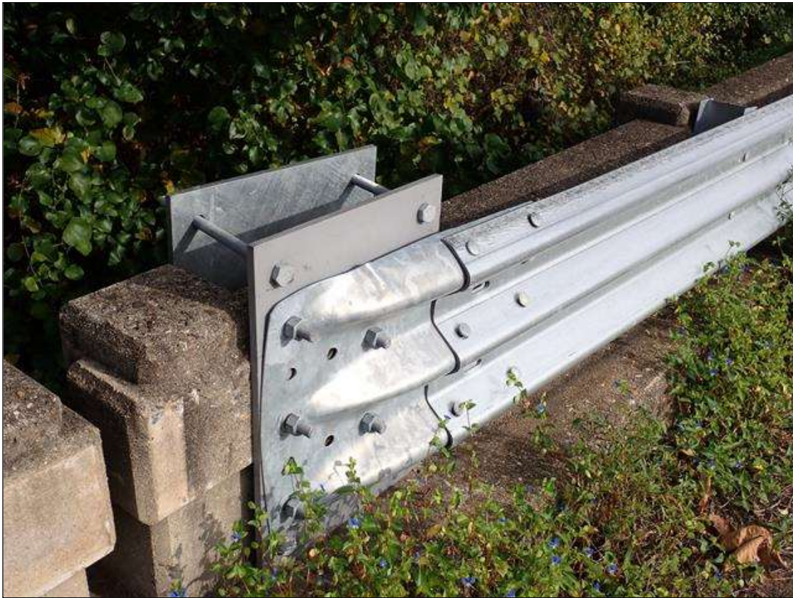
(PAR) northwest guardrail attachment, (2) bolts missing
