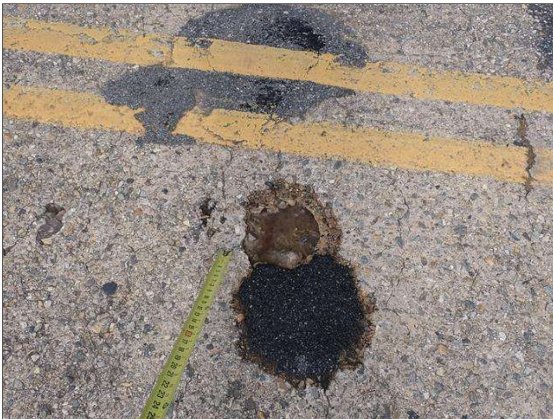
Span 4 Deck: (PAR) throughout top of deck, scattered delaminations/spalls (up to 1 foot diameter x 1.5 inch deep), some with exposed rusted rebar
