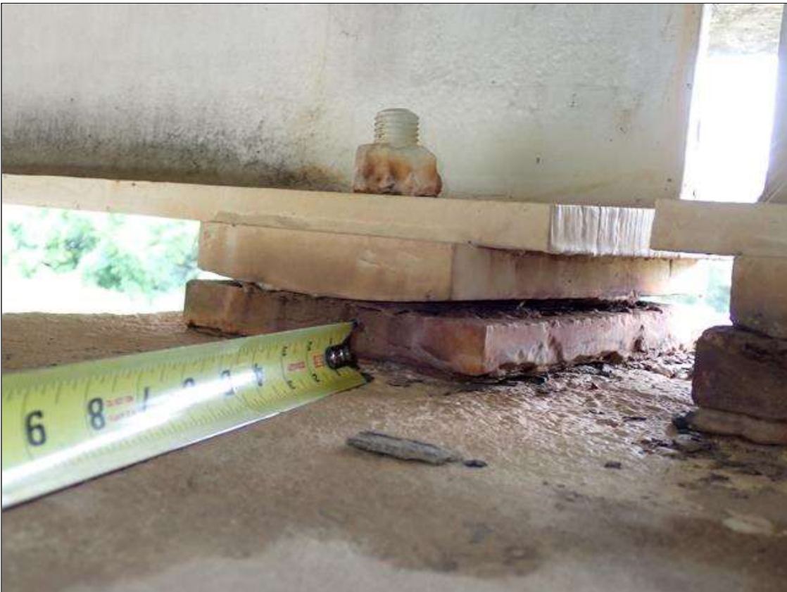
Span 2 Beam 4 - Near Bearing 4: painted over section loss (up to 1/8 inch deep) with corrosion reinitiated
