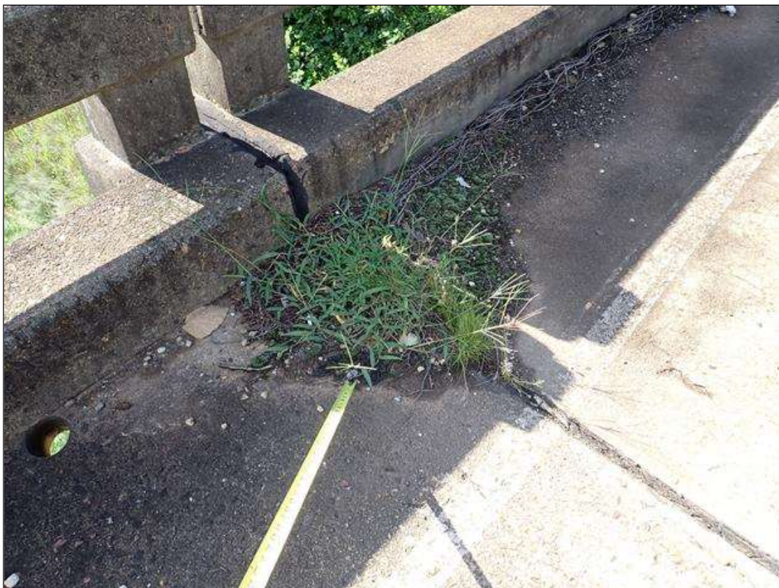
Span 2 Bent 1 Joint: both shoulders, debris accumulation
