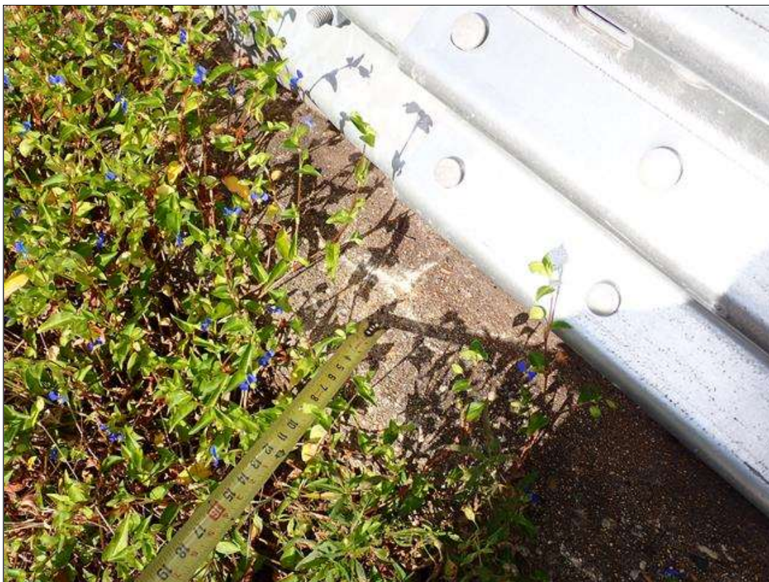
Span 4 Left Bridge Rail: along the curb, areas of map cracks (hairline) at random, some with efflorescence
