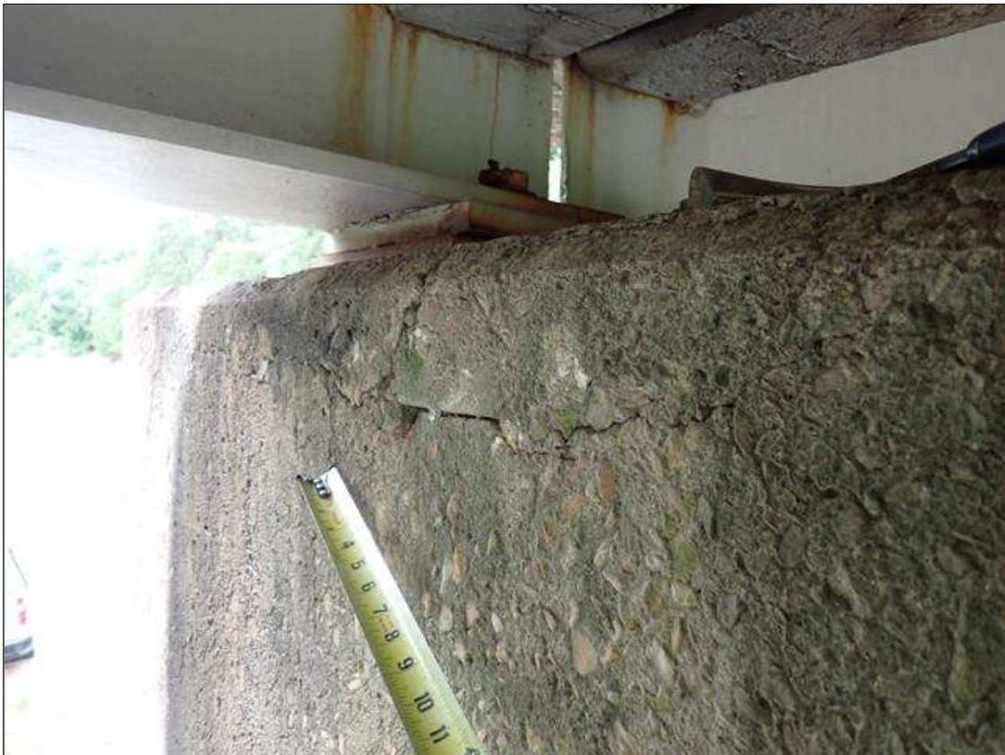
Bent 2 Cap 1: south and north faces, and underside, delaminations (up to 5 feet x 6 inch) with associated longitudinal cracks (up to 1/16 inch); areas of map cracks (hairline) at random
