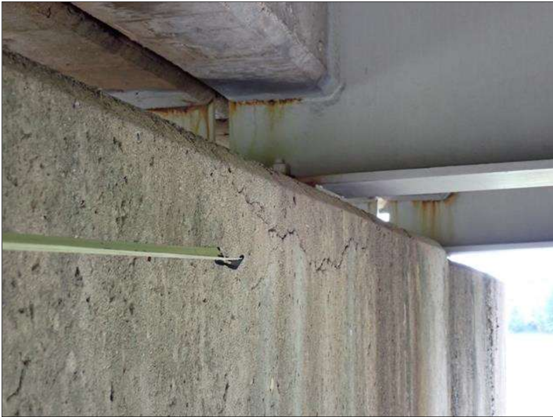
Bent 2 Cap 1: south and north faces, and underside, delaminations (up to 5 feet x 6 inch) with associated longitudinal cracks (up to 1/16 inch); areas of map cracks (hairline) at random
