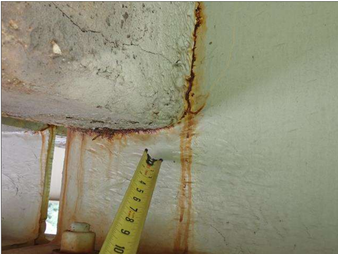
Span 1 Beam 2: at bent 1, web adjacent to diaphragm, painted over section loss (7/16 inch average remaining x 7 inch x 4 inch) with corrosion reinitiated
