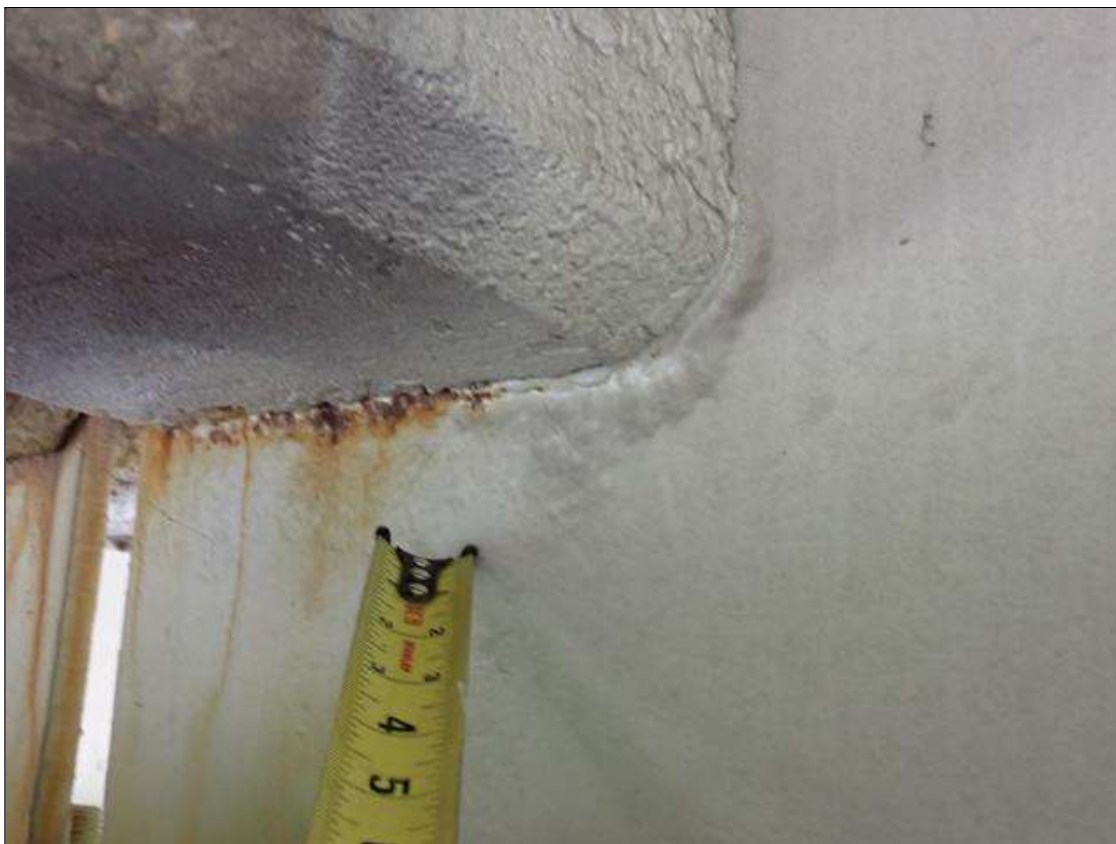
Span 2 Beam 3: at bent 2, web adjacent to diaphragm, painted over section loss (7/16 inch average remaining x 7 inch x 1.5 inch) with corrosion reinitiated
