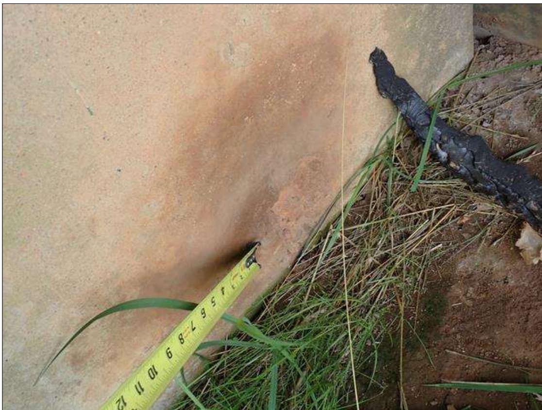
Bent 1 Pile 1: east face, at ground, spall (5 inch x 4 inch x 1 inch deep)
