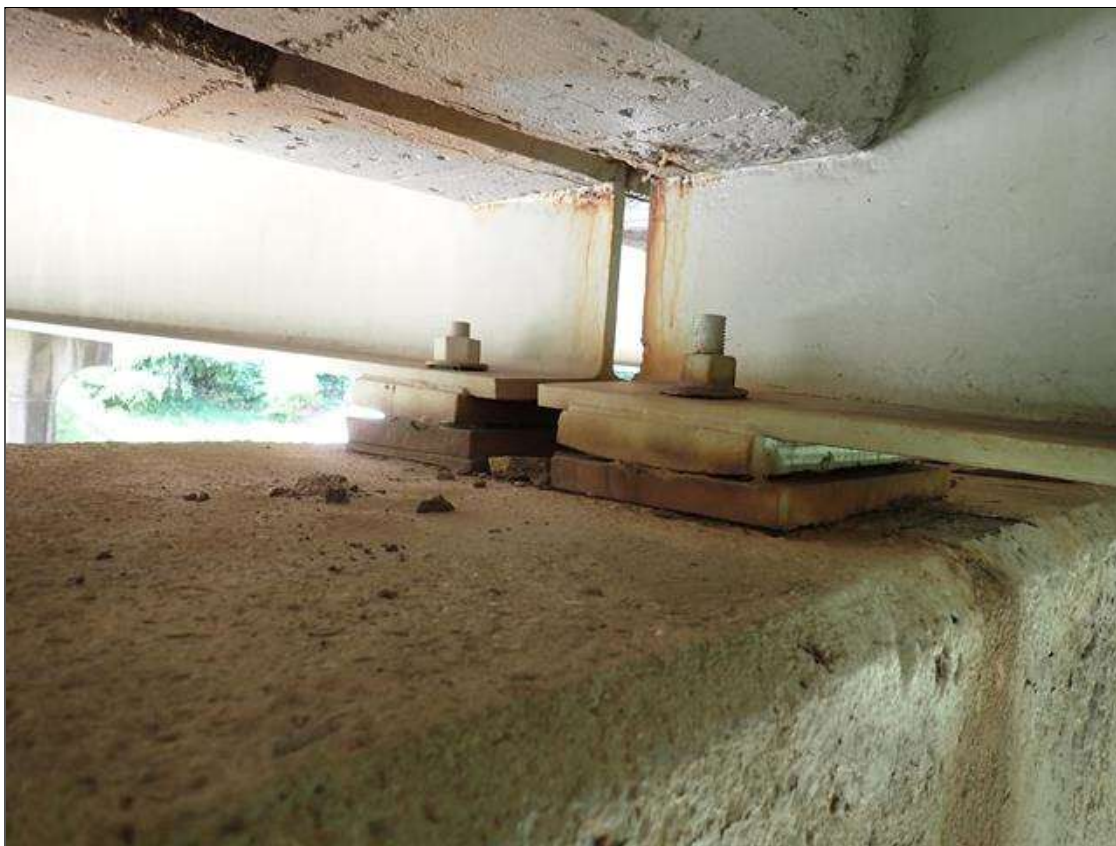
interior bearing assembly
