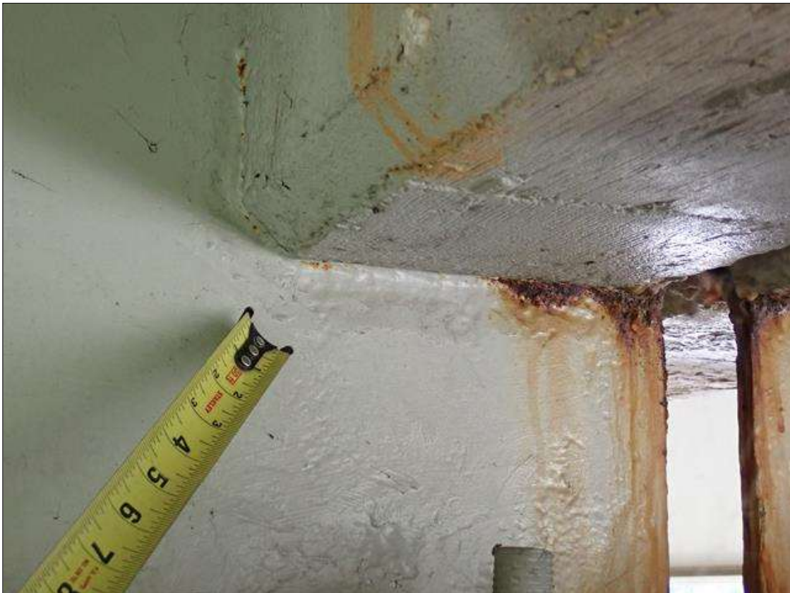
Span 4 Beam 2: (PAR) at bent 3, web adjacent to diaphragm, painted over section loss (5/16 inch average remaining x 9 inch x 2 inch); lower web, painted over pitting (up to 1/8 inch deep x 6 inch x 6 inch) with corrosion reinitiated
