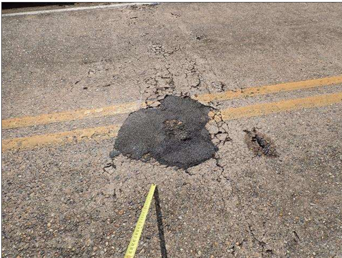
Span 3 Deck: 2 - TOP OF DECK HAS ASPHALT PATCHED AREAS ALONG THE CENTER LINE UP TO 2.5 FEET X 3 FEET.
