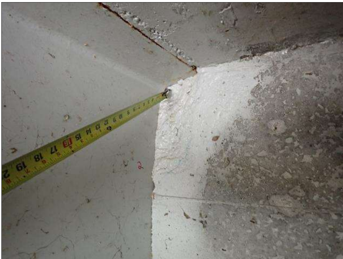
End Bent 2 Abutment: in bay 2 adjacent to East face of beam 2, spall [5 inch x 11 inch x up to 1.5 inch deep]
