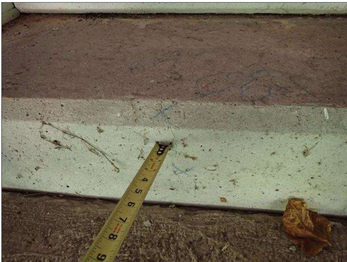
End Bent 2 Abutment: along length of cap, multiple vertical cracks [up to full height x 1/64 inch]
