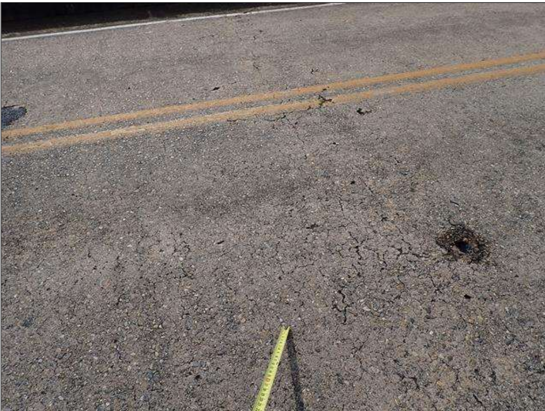
Span 3 Deck: throughout top of deck, map cracks (up to 1/16 inch) and transverse cracks (up to 1/16 inch x 15 feet) at random
