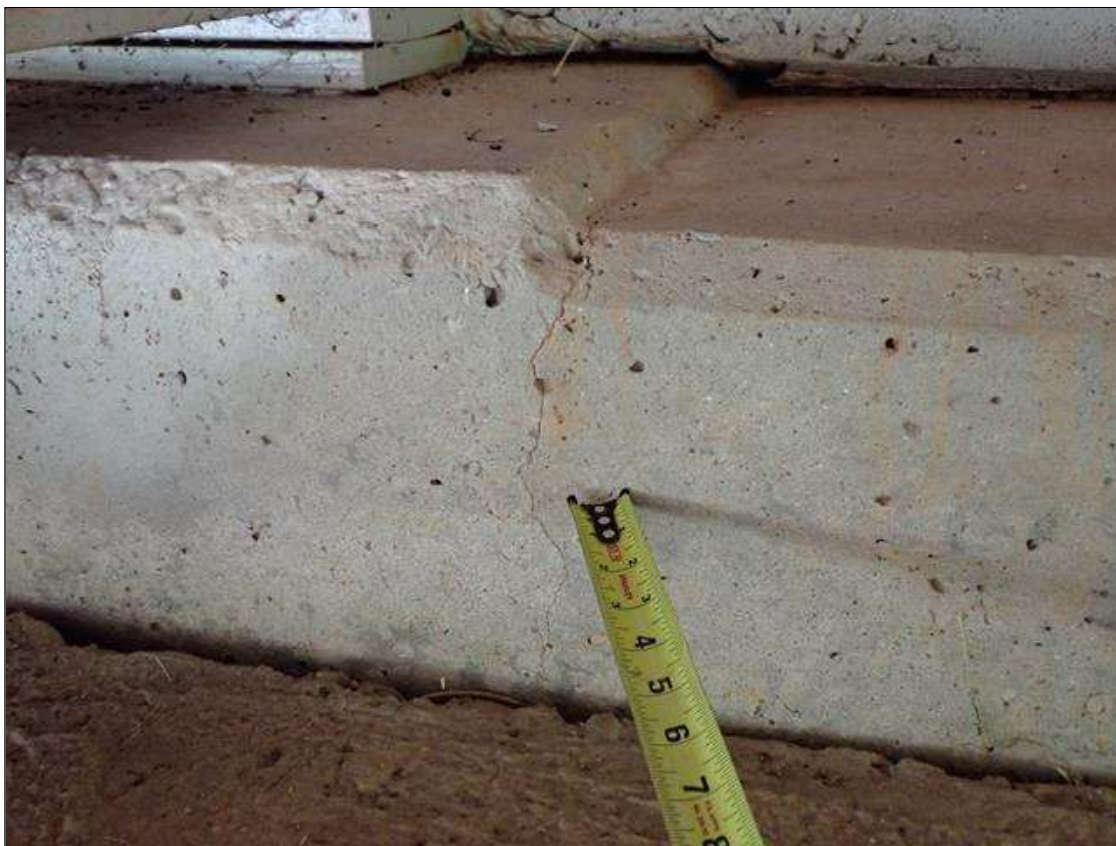
End Bent 1 Cap 1: along length, multiple vertical cracks [up to full height x 1/32 inch]
