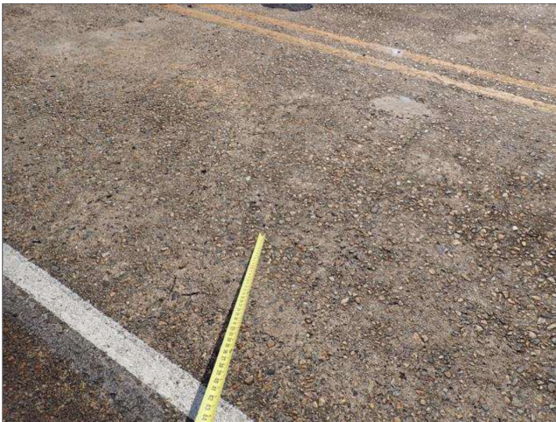
Span 2 Deck: throughout top of deck, wear with secure aggregate
