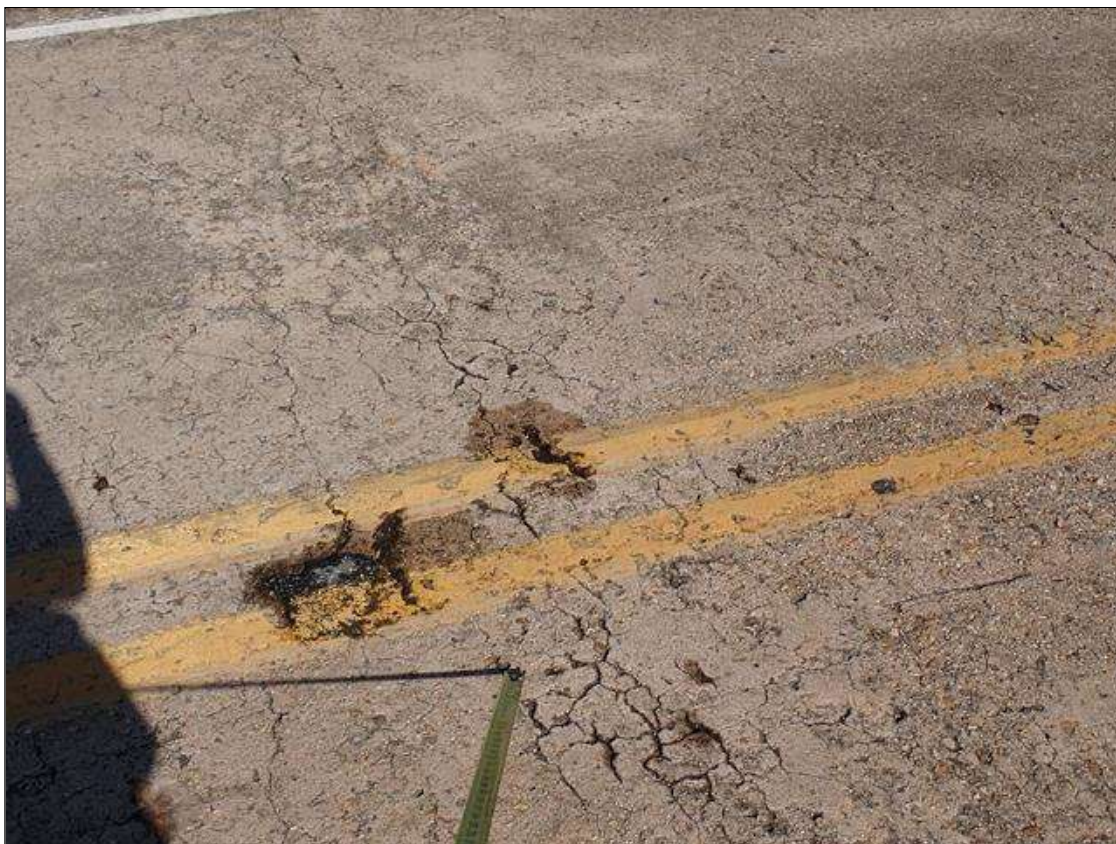
Span 1 Deck: (PAR) throughout top of deck, scattered delaminations/spalls (up to 2 foot x 1 foot x 1.5 inch deep), some with exposed rusted rebar
