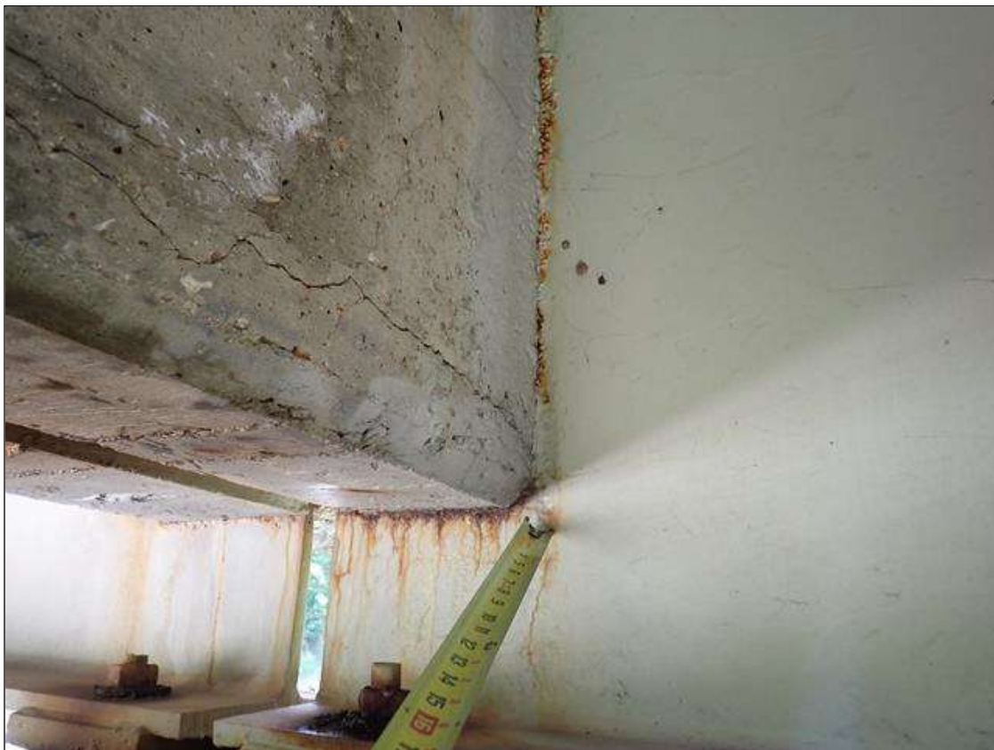
Span 4 Beam 1: at bent 3, web adjacent to diaphragm, painted over section loss (7/16 inch average remaining x 9 inch x 2 feet) with corrosion reinitiated
