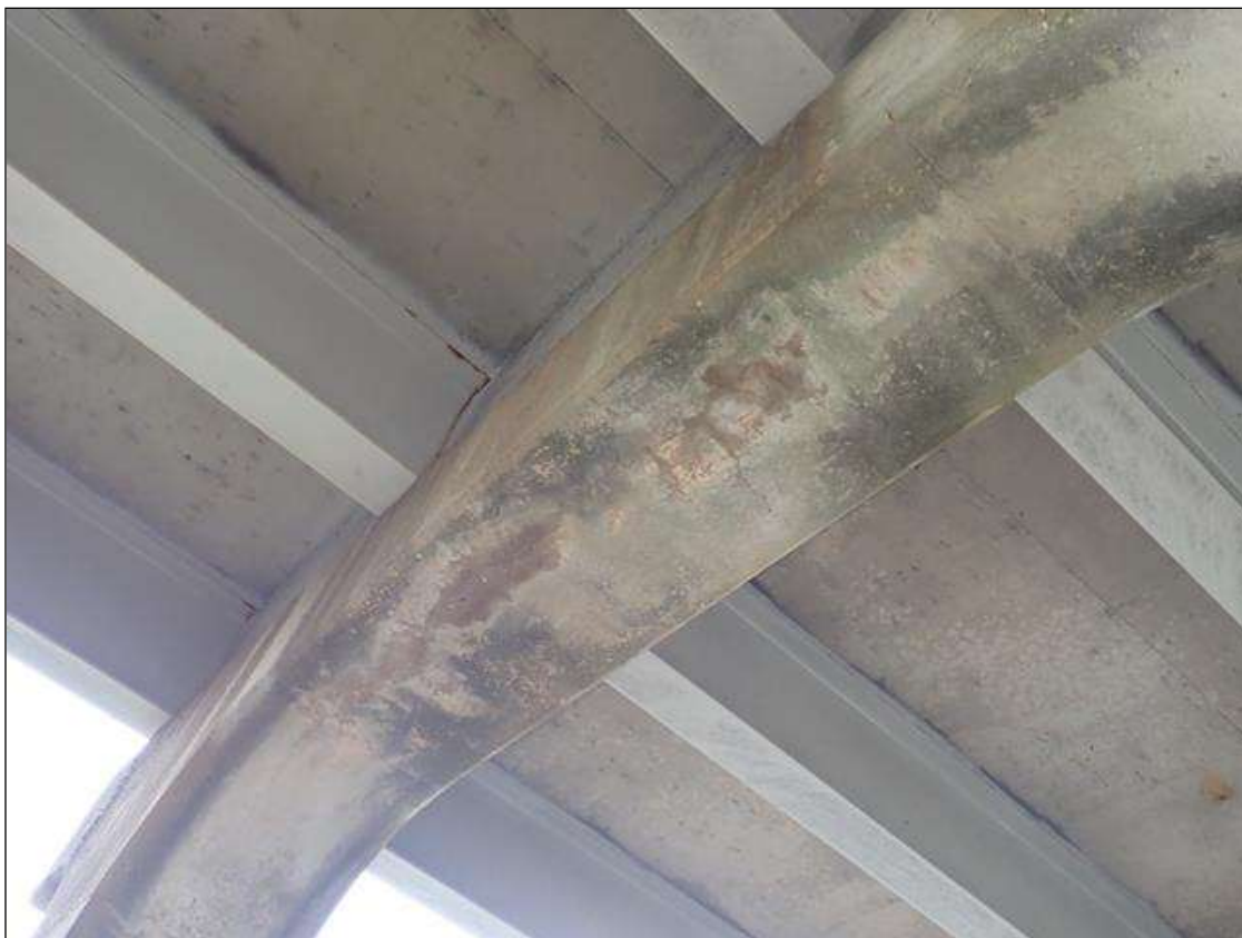
Bent 2 Cap 1: south and north faces, and underside, delaminations (up to 5 feet x 6 inch) with associated longitudinal cracks (up to 1/16 inch); areas of map cracks (hairline) at random
