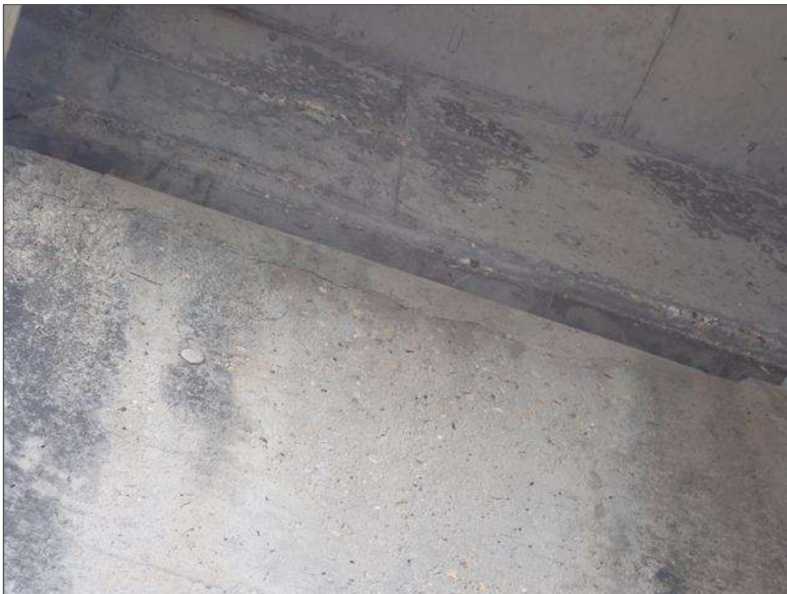
Bent 1 Cap 1: along the length of the cap, delaminations (up to 7 feet x 6 inch) with cracks (up to 1/16 inch)
