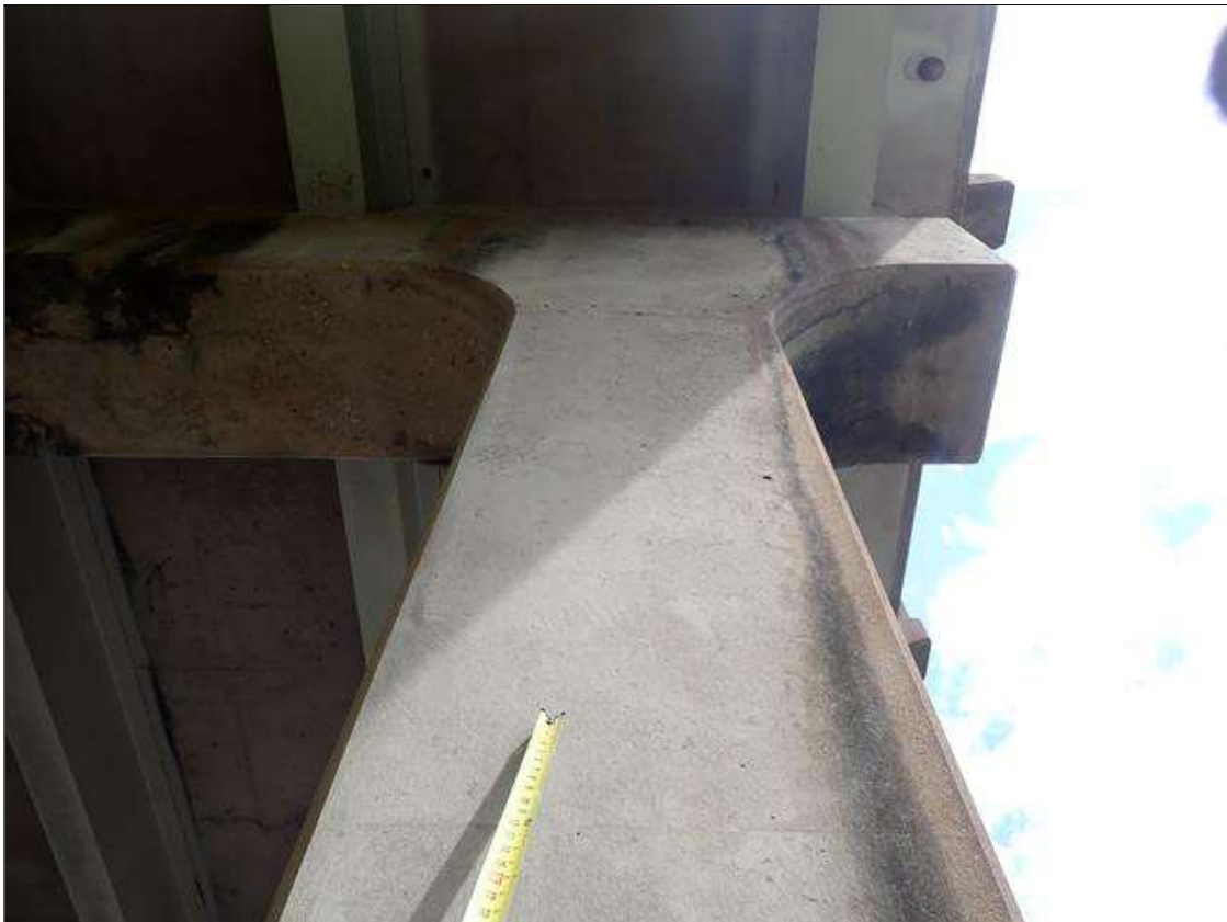
Bent 1 Pile 2: all faces, vertical cracks (up to 1/32 inch x 7 feet) and areas of map cracking (hairline) at random
