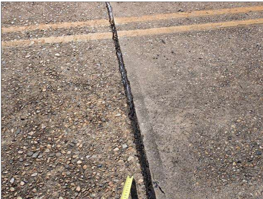
Span 2 Bent 1 Joint: along the length of the joint, deteriorated seal at random
