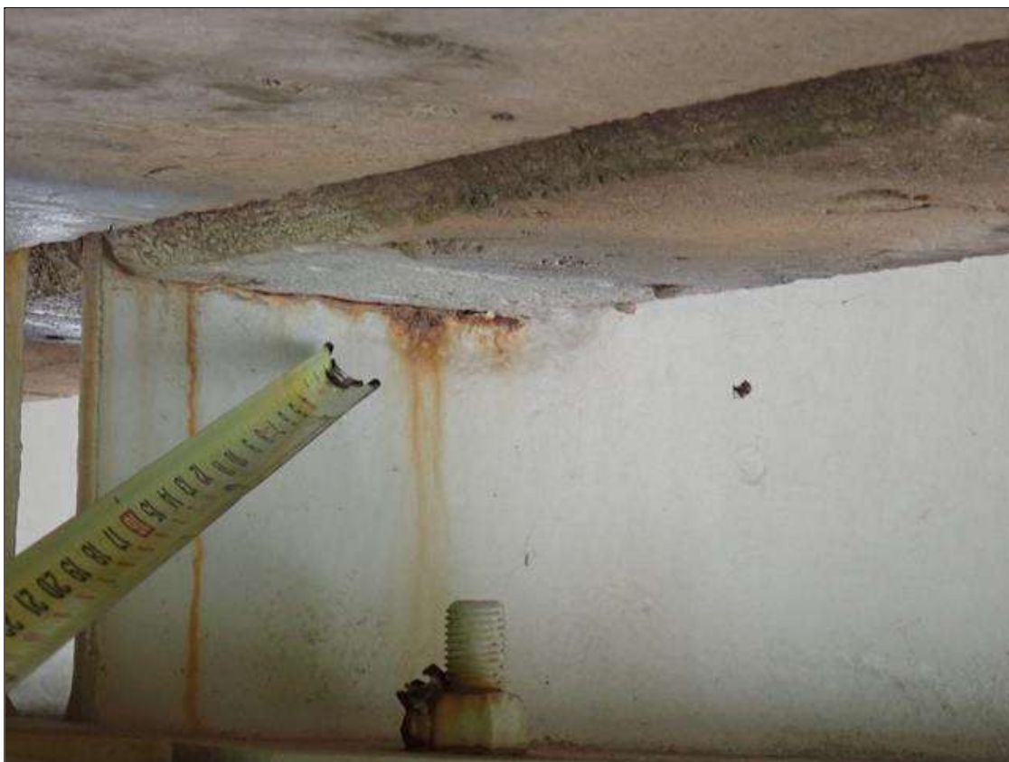
Span 3 Beam 3: (PAR) at bent 2, web adjacent to diaphragm, painted over section loss (3/8 inch average remaining x 10 inch x 1 inch) with corrosion reinitiated
