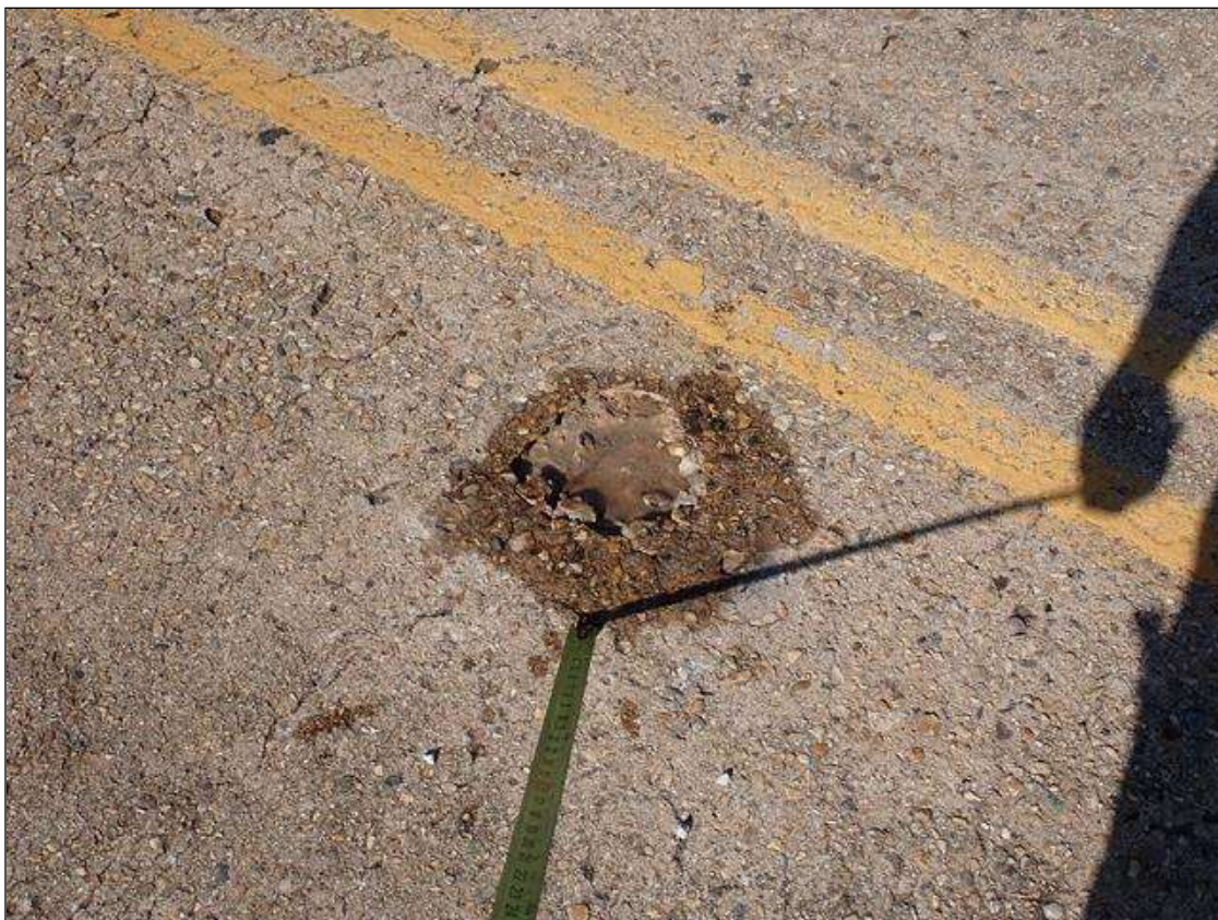
Span 1 Deck: (PAR) throughout top of deck, scattered delaminations/spalls (up to 2 foot x 1 foot x 1.5 inch deep), some with exposed rusted rebar
