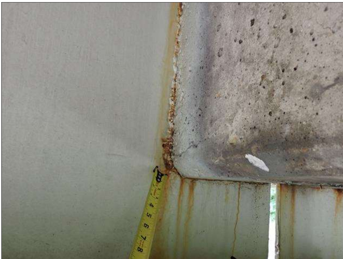
Span 2 Beam 1: at bent 2, web adjacent to diaphragm, painted over section loss (1/2 inch average remaining x 1 inch x 6 inch) with corrosion reinitiated
