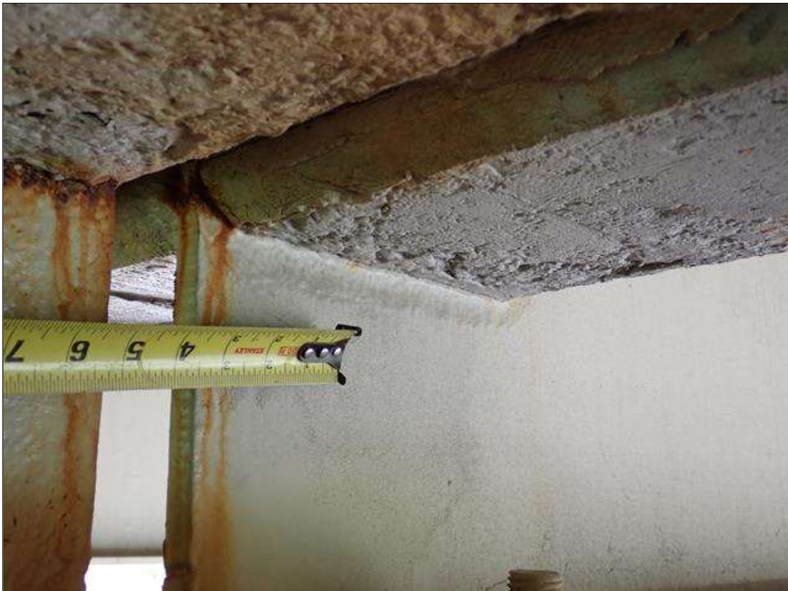
Span 2 Beam 2: (PAR) at bent 1, web adjacent to diaphragm, painted over section loss (3/8 inch average remaining x 10 inch x up to 2 inch) with corrosion reinitiated
