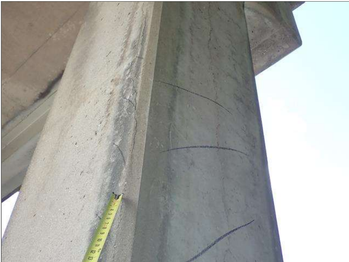
Bent 3 Pile 1: 7 FOOT X UP TO 1/16 INCH VERTICAL CRACKS ON EAST, WEST AND NORTH FACES AT BOTTOM OF CAP with associated delamination [5 feet x 2.5 feet]
