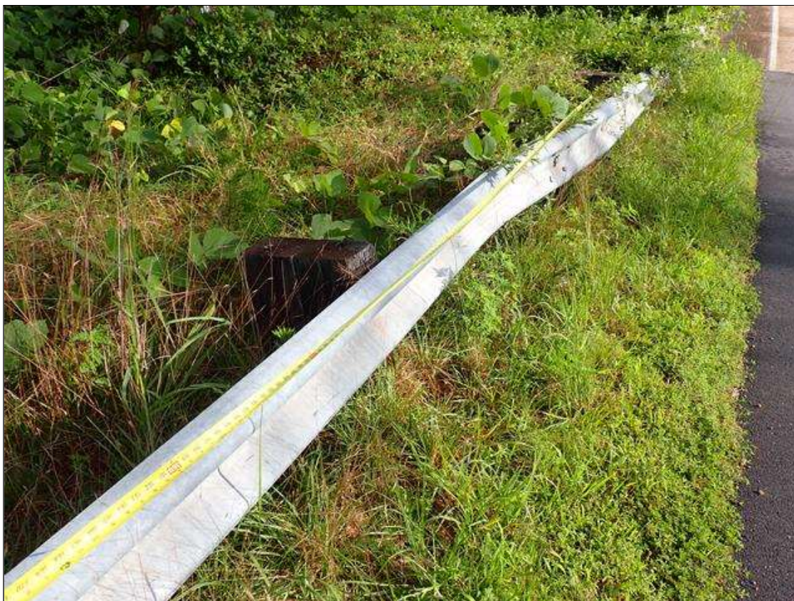
(PAR) southwest guardrail, approximately 15 feet from bridge, impact damage (15 feet)
