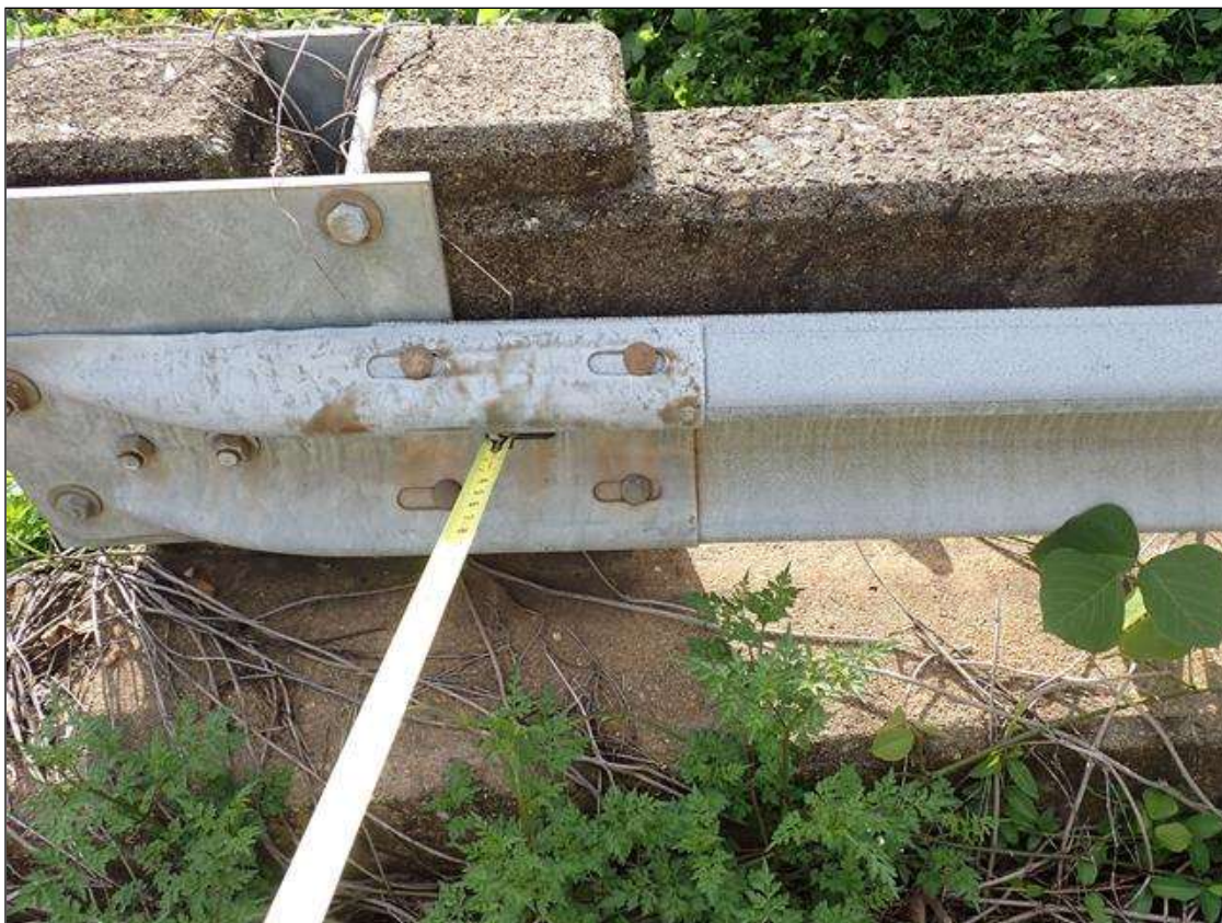
(PAR) southeast guardrail attachment, improper lap
