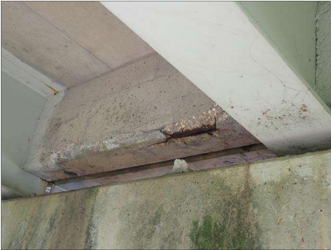
Span 1 Deck: at bent 1, end diaphragm in all bays, spalls/delaminations (up to full bay width x 6 inch wide x 15 inch deep) with exposed rusted rebar and associated cracks (up to 1/16 inch)
