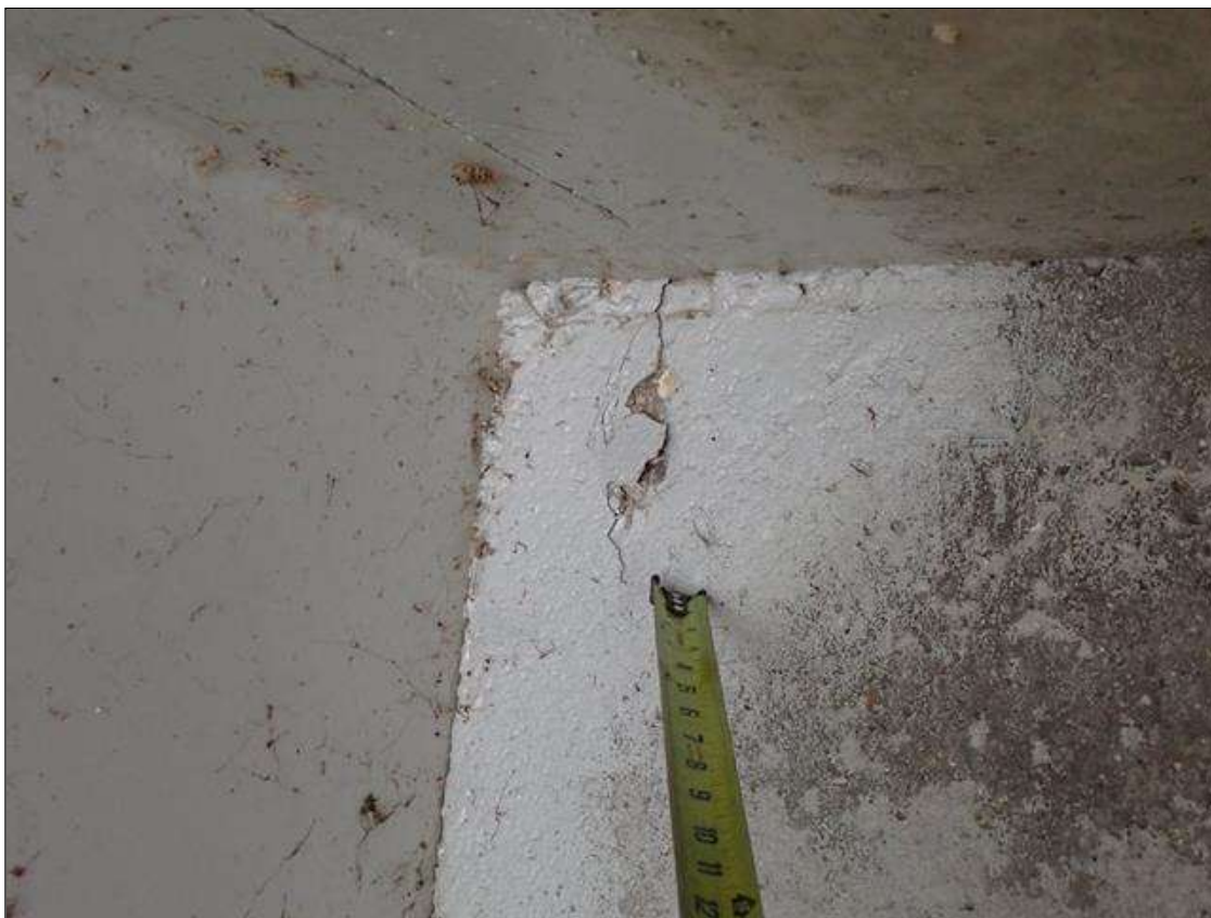
End Bent 1 Abutment: adjacent to all beams, delaminations/spalls [up to 2 feet x 13 inch x 1/2 inch deep]
