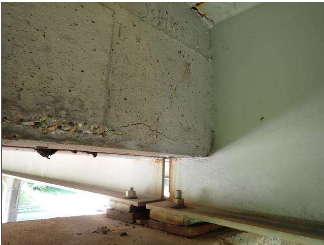
beams over bent
