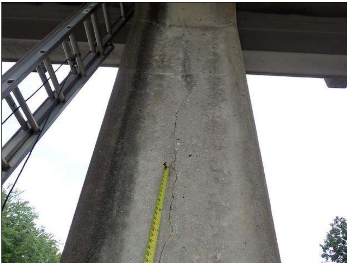
Bent 2 Pile 1: UP TO 11 FOOT X UP TO 1/16 INCH VERTICAL CRACKS ON EAST AND WEST FACES.
